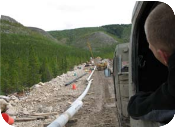
Rigorous Terrain – minimize traffic in extreme elements, in and out of site
