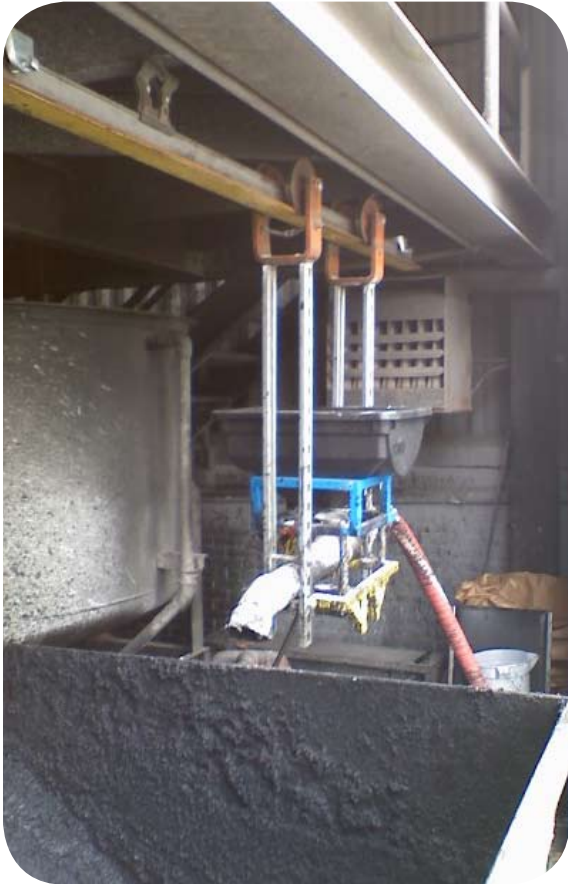
LiquiSorb feeder mounted on overhead monorail
