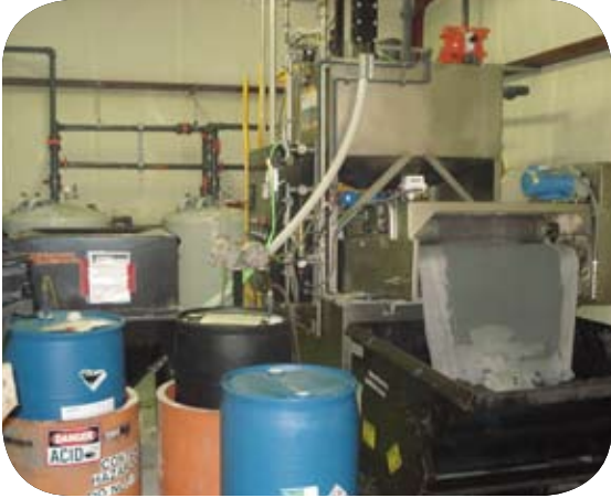
CE-200GA Unit in Action Treating All Plant Wastewater
