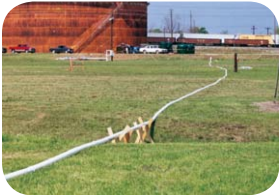
The pipeline constructed to transfer treated water from CETCO's equipment to the stream.
