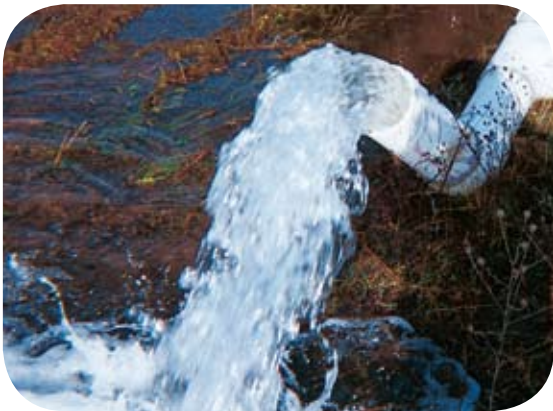
Clean Water Discharge Point
