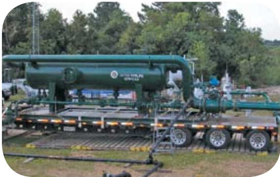
High Pressure Separator
