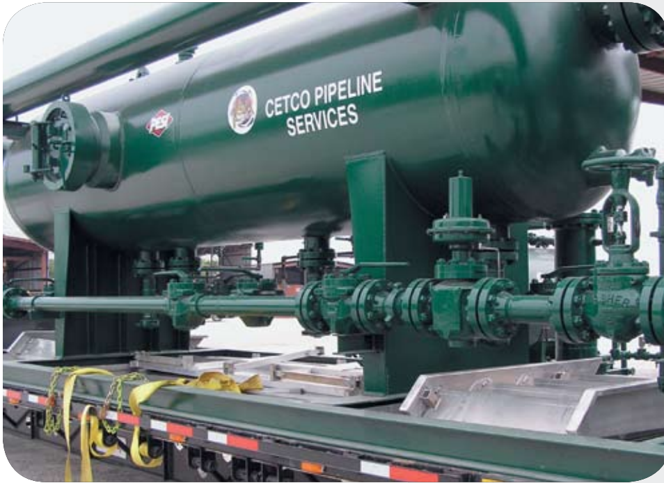
High Pressure Separator
