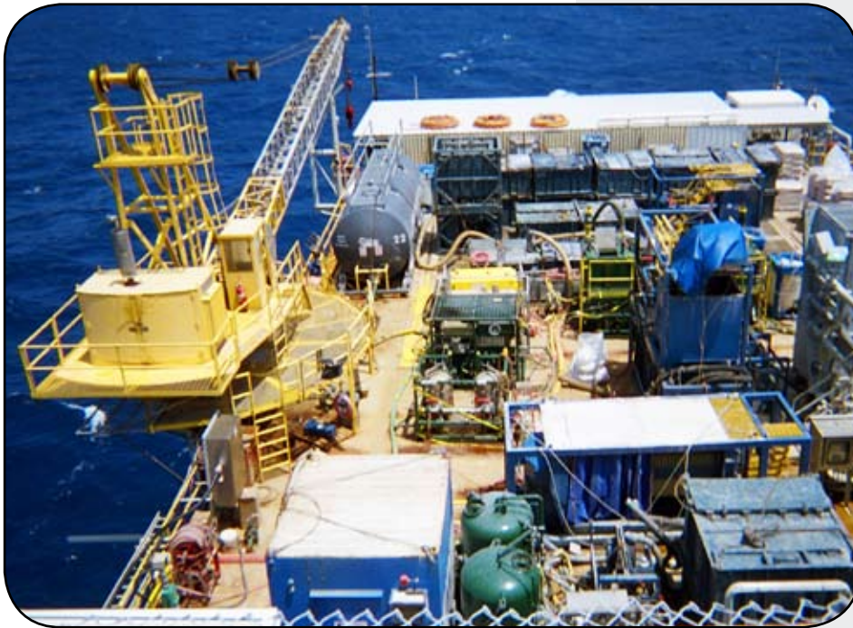
Customer's offshore production platform with customer's, CETCO's, and 3rd party's production treatment equipment
