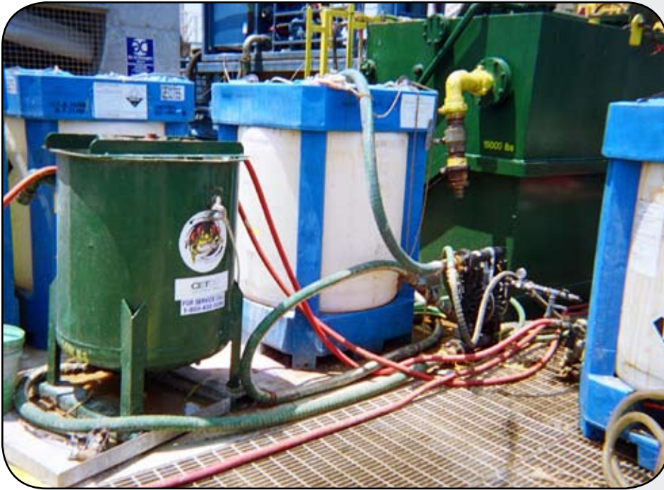
Produced water chemical treatment setup
