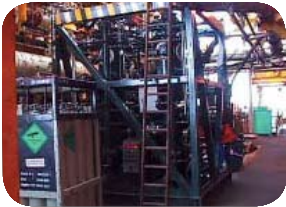
CETCO equipment on Auk platform
